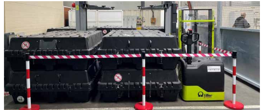
Batteries storage on the floor
