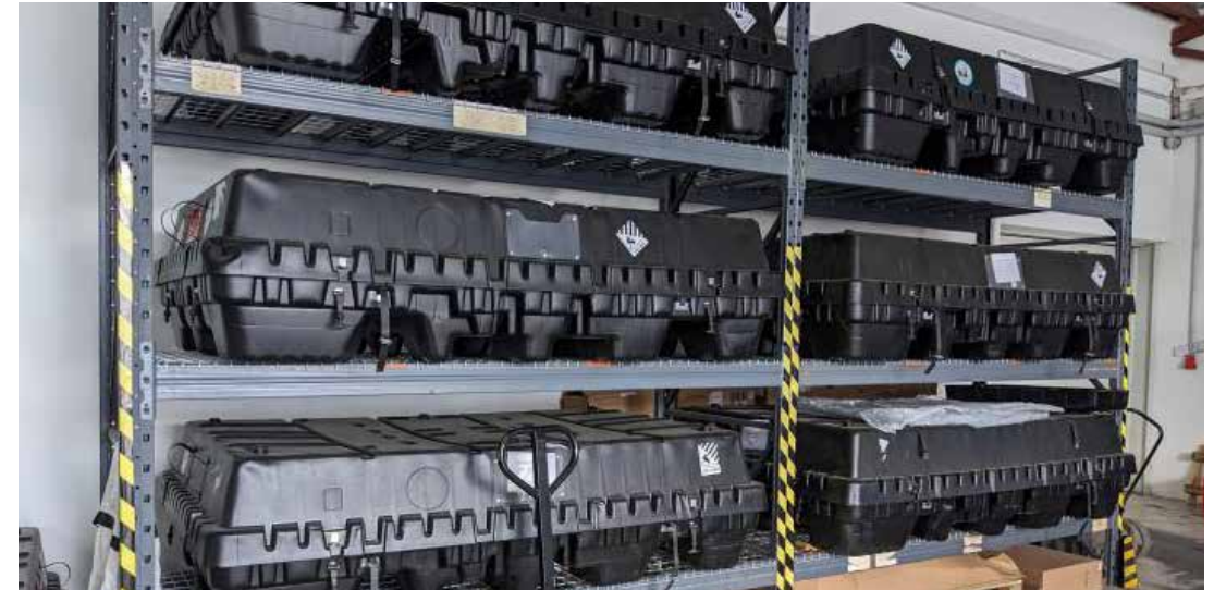
Batteries storage on rack
