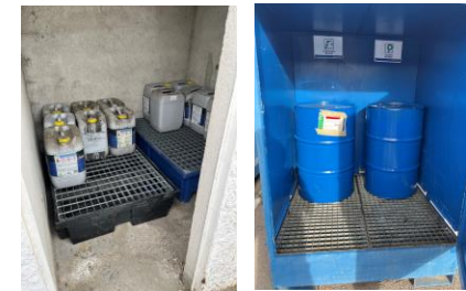
Outdoor storage of hazardous waste
